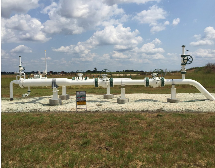
Gathering line system in the Eagle Ford area
